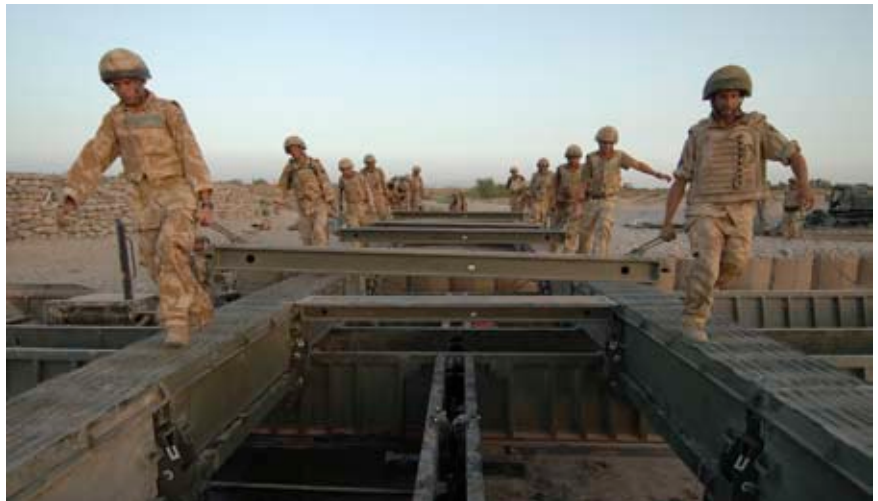
In an operational engineering first, engineers lay an air portable ferry bridge across the River Helmand in just seven hours
